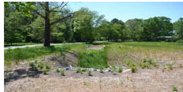
This structure captures all the water that flows through the open channel swale as well as runoff from the rear entrance. It's primary features are an underdrain system that allows greater infiltration of stormwater and vegetation to treat and purify runoff before discharge to a stream.
