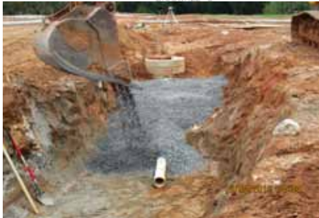
A perforated underdrain and gravel bed allows water to infiltrate back into the groundwater table.
